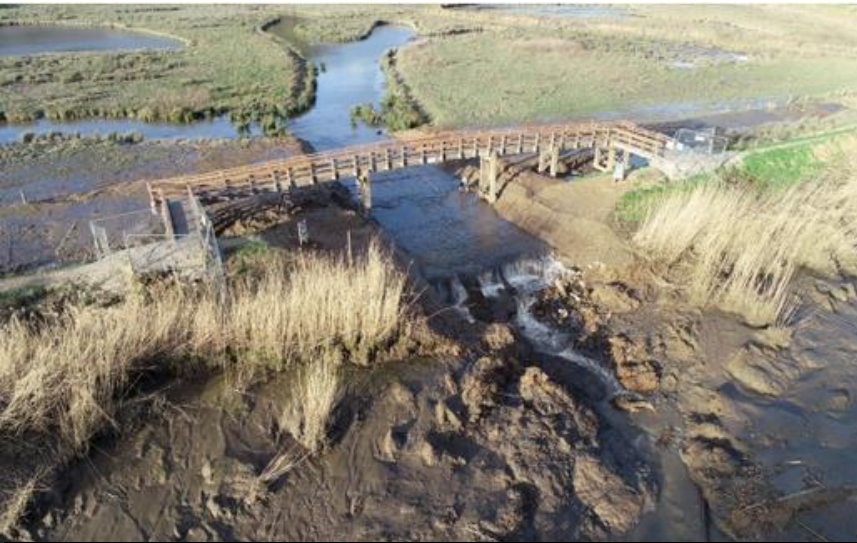
A bridge over the breach in the flood bank at Calstock flood defence improvement scheme, Jan 2022. Photo: Will Jay, Airborne Earth Observation Data Analyst at PML
