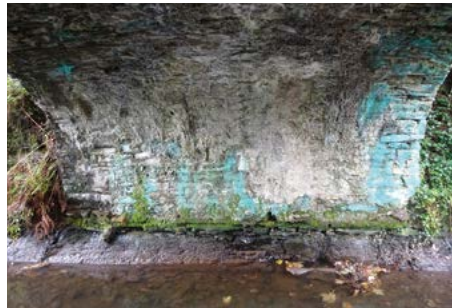
Copper staining under Crowndale Bridge
